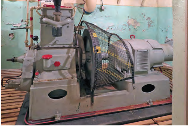
Standby generator near the entrance of the Csepel Command Centre
